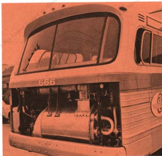
The steam generator assembly is installed in original diesel engine compartment at rear of bus. Automatic controls govern flow of fuel and water.
